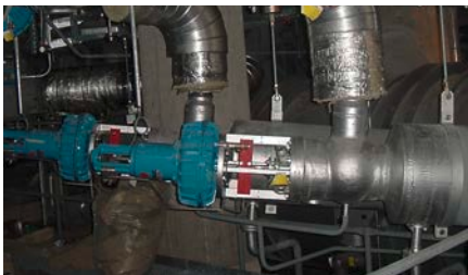
Turbinen-Bypass-Station Turbine Bypass Station
