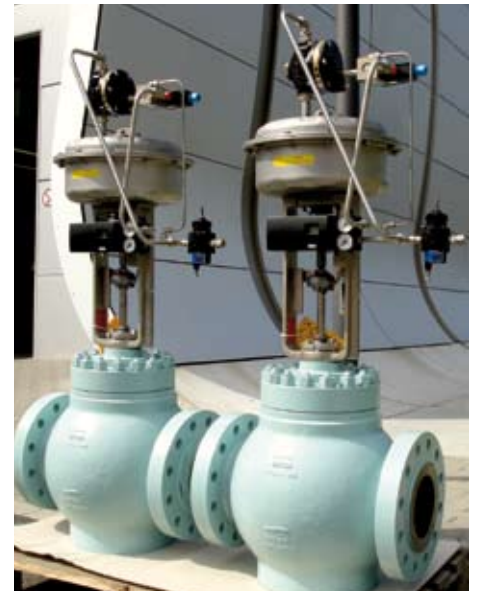
Abb.: N 2 -Verdichter Bypass-Ventile ▲ Picture: N 2 compressor bypass valves ▲
