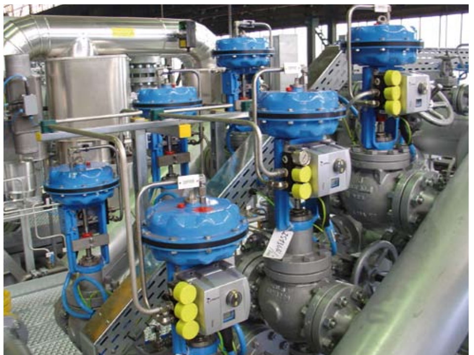
Picture: Valves in operation at a PSA-skid plant ▼
